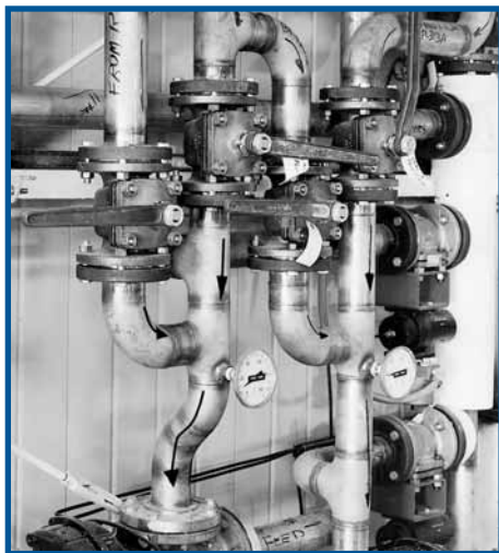
Flowserve McCannaSeal valves in steam application
