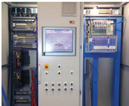
SIL-2 PLCs with interactive touch-screen color HMI and BN monitoring systems inside a control room
