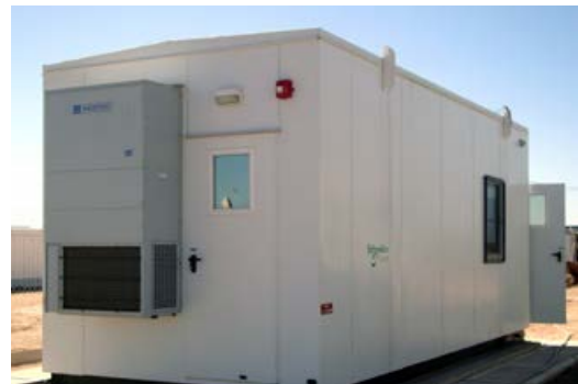
Fully equipped power house with switchgear, PLCs, HVAC, and fire and gas system to control and operate two MP1-380 units in Argentina
