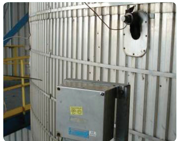
High-temperature accelerometers monitor vibrations on the coke drum wall. The resulting signals provide the operator with information regarding drum cleanliness status.
